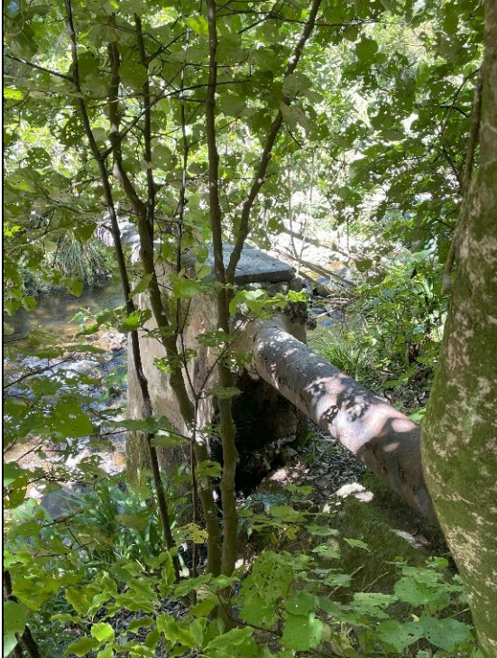
Figure 4.5: Leaking sewage pipe in Trelissick Park.
