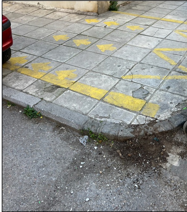
Figure 4.7: Missing Curb Ramp and Tactile Slab on the Corner of Cheiokratous and Vithynias
