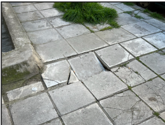
Figure 0.3: Cluster of Broken Sidewalk Tiles on Michail Chourmouz
