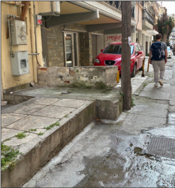
Figure 0.2: Sidewalk with Step and Blockage on Vithynias Street (near SFA center)
