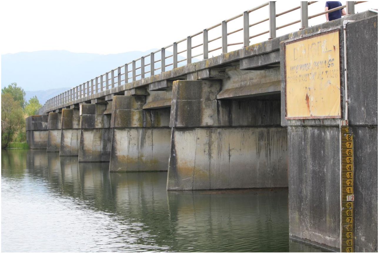
Figure 14 - The Blundell Barrage Gates: side view
